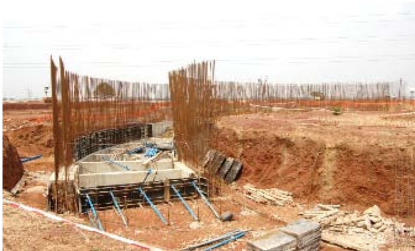
SINTER COOLER AREA
