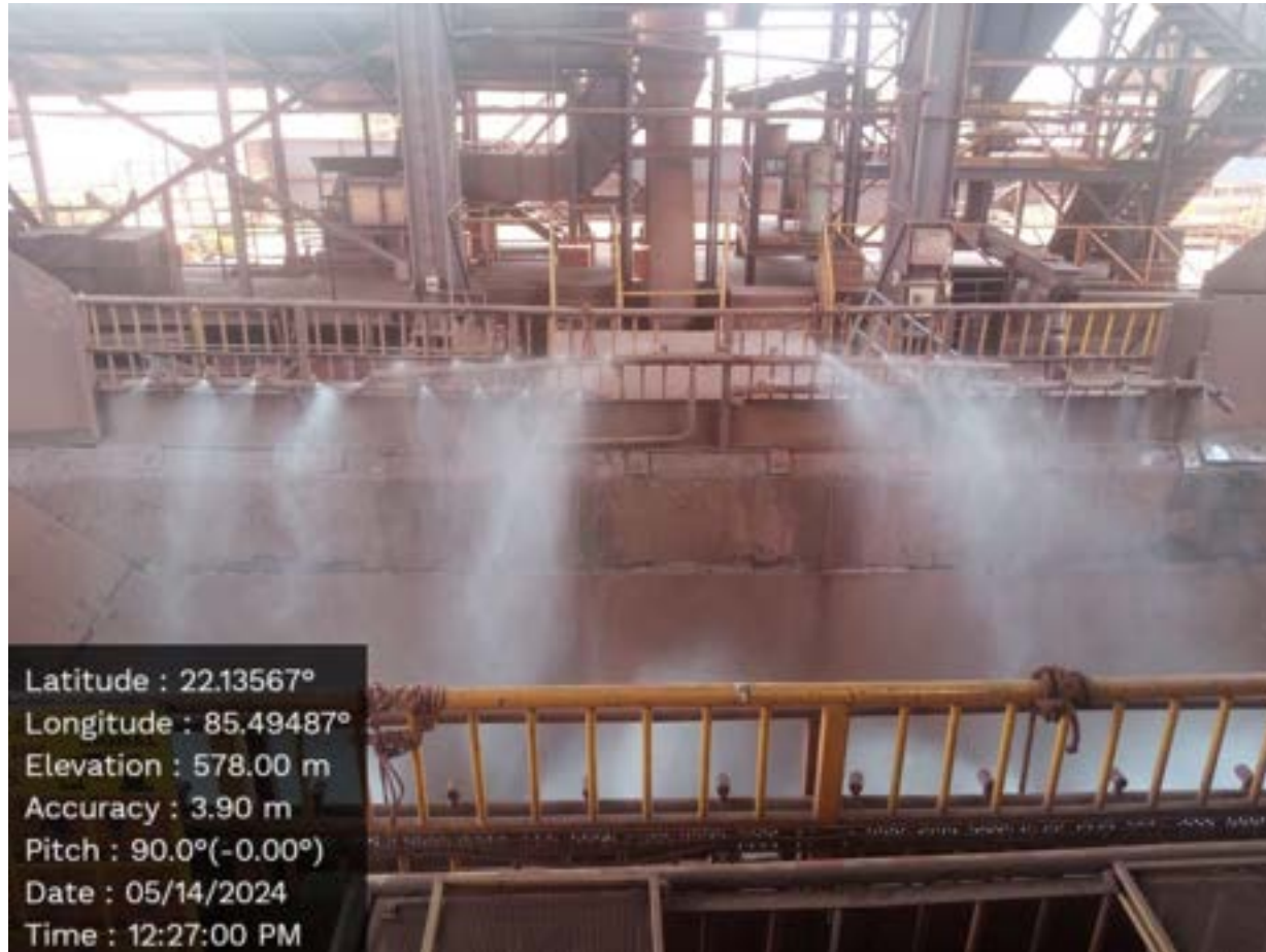
Dry-fog system installed at Crushing & Screening Plant
