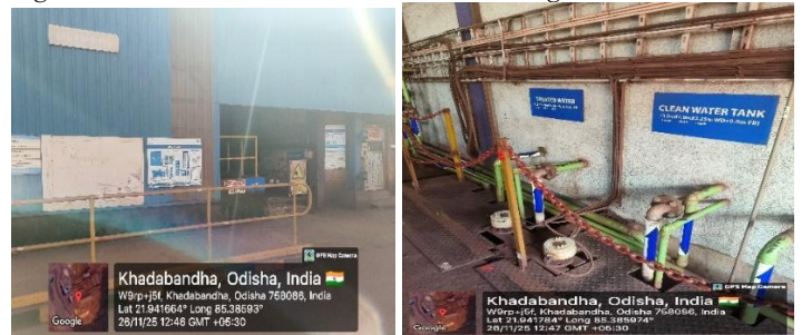
Fig 22: 7 KLD ETP at Khondbond Iron and Manganese Mine
