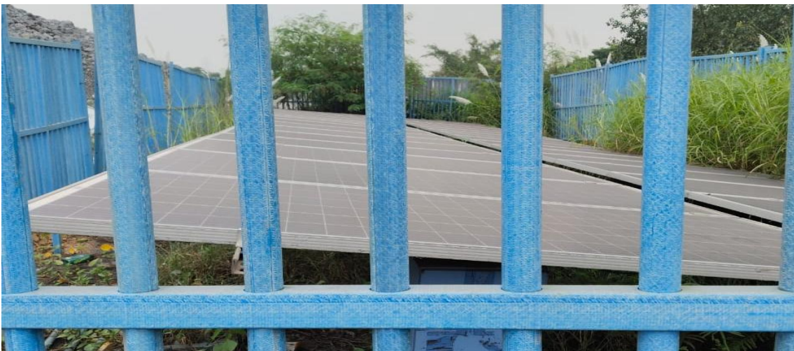
(Solar power panel installed at TSM)
