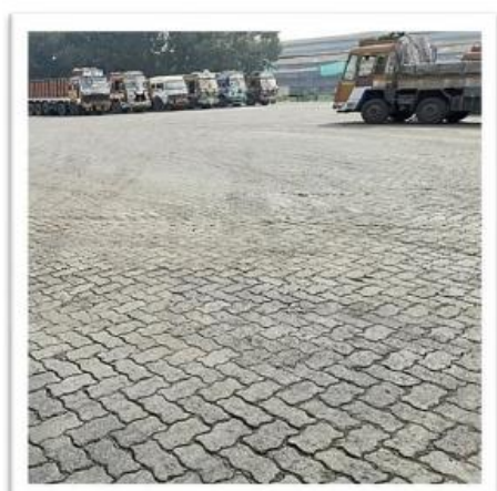
Paver Blocks on loose soil
