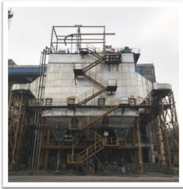
Electrostatic Precipitator (ESPs) at Boiler Stack
