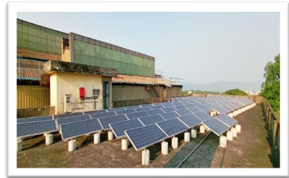
Solar panel at Cold Rolling Mill
