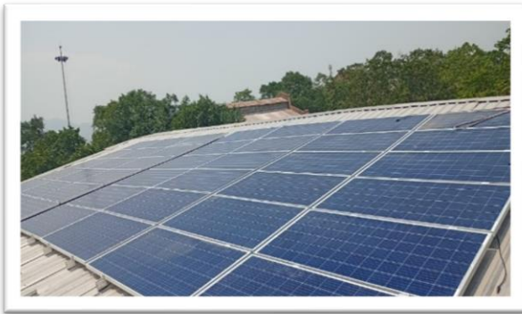
Solar panel at Printing & Lacquering Line
