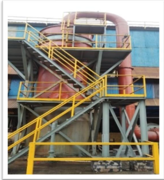
Scrubber at Pickling
