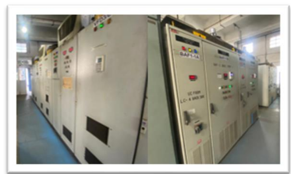
Variable Frequency Drive for all Mill and process line motors
