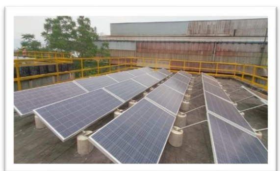
Solar panel at Coil Preparation Line
