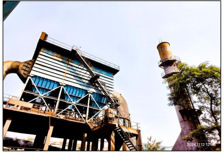
Adequate APCS have been Installed at different
