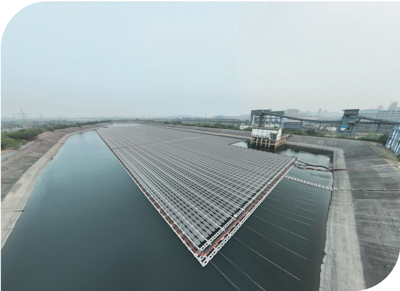
Solar Plant on Water Reservoir, Tata Steel Kalinganagar
