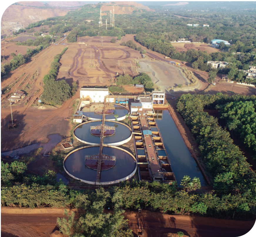
Water Treatment Plant, Meramandali
