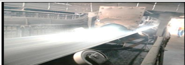
Dust Suppression system at Transfer points
