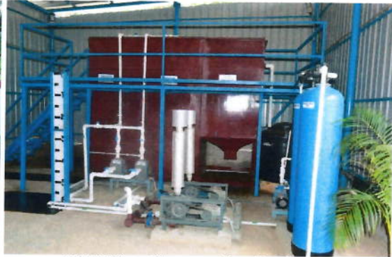
10KLD Effluent Treatment Plant (ETP) at Hospital
