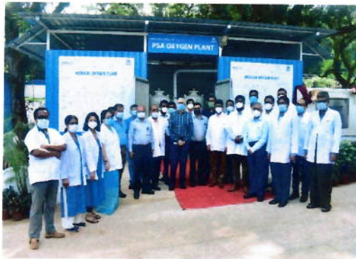
PSA Oxygen Plant installed at TSH-Noamundi
