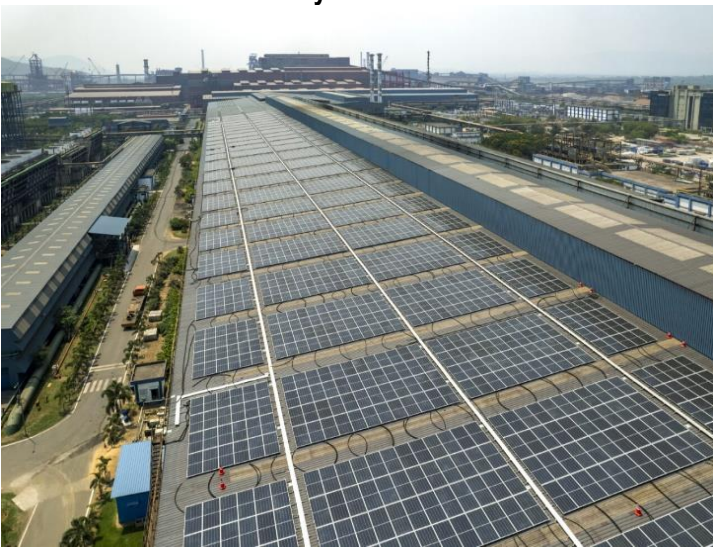
PV Solar Panel installed at HSM Roof top
