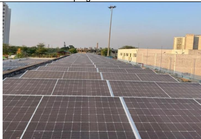
Solar Panels installed at roof top of Buildings
