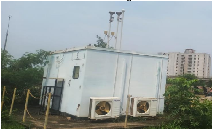
Continuous Ambient Air Quality Monitoring Station
