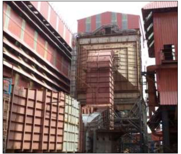
De-dusting ESP at Blast Furnace
