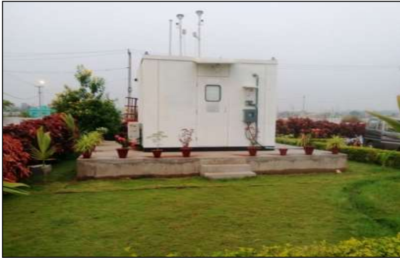
Continuous Ambient Air Quality Monitoring Station
