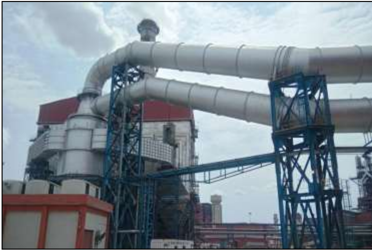
Cyclone and ESP installed at SMS
