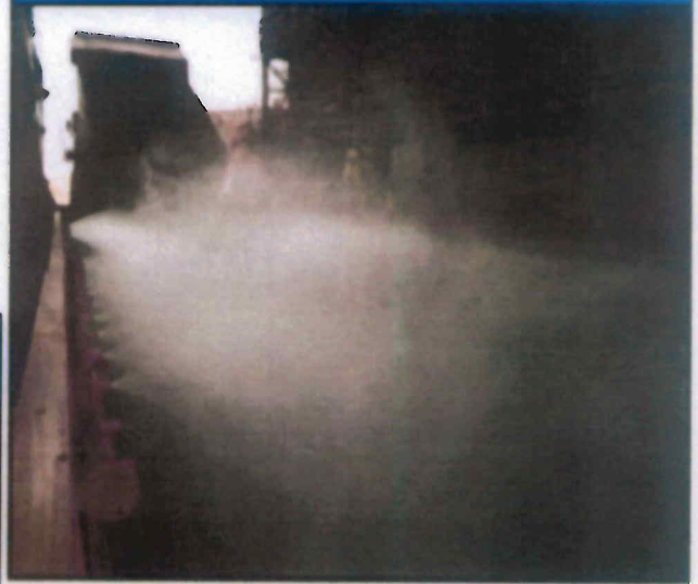
Water Jet system at Primary Crusher
