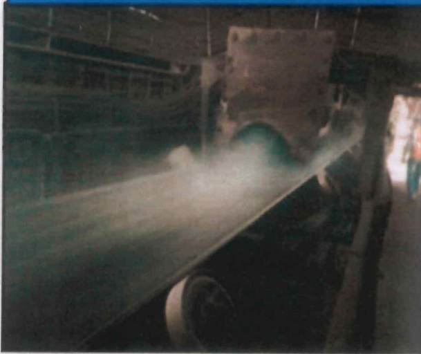
Dry fog system in plants
