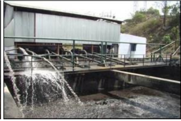
Effluent recycling in washery
