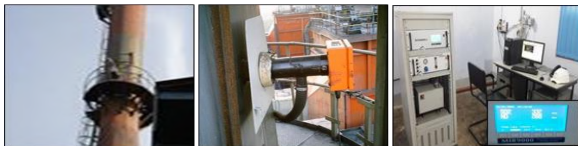
Continuous Emission Monitoring for Power House for PM, Sox & NOx data
