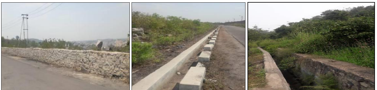
Toe wall & garland drain in the area
