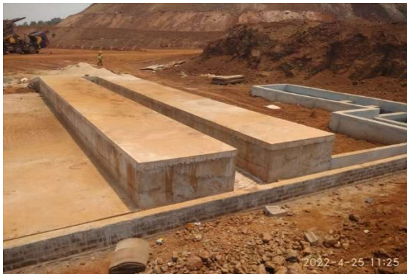
Vehicle washing with Oil & Grease separation pit
