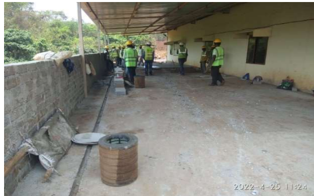
Hazardous storage area
