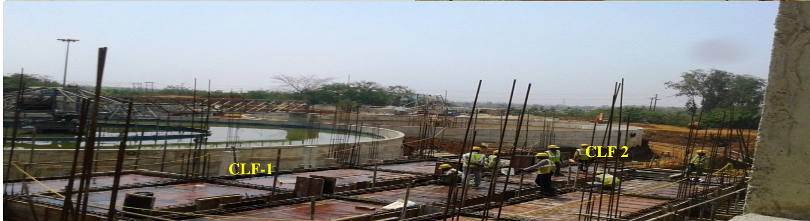
Clariflocculator of New ETP
