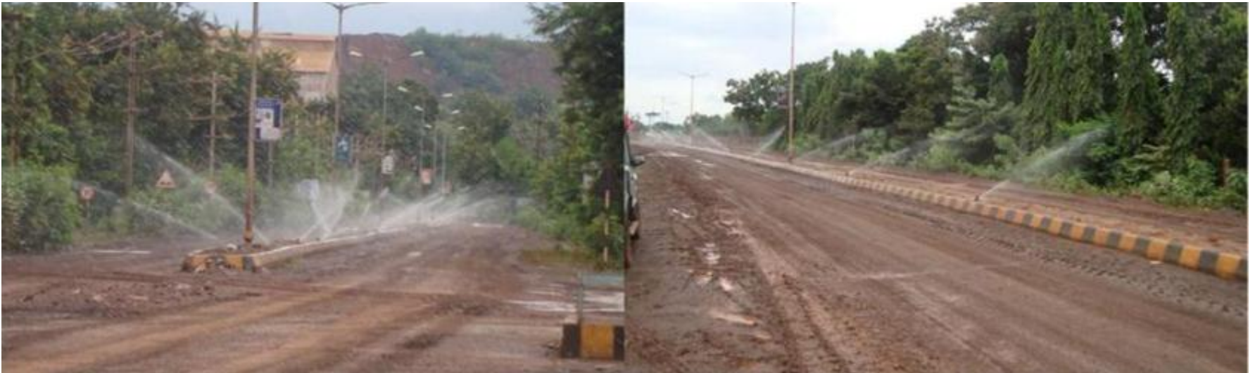
Stationary Water Sprinkler
