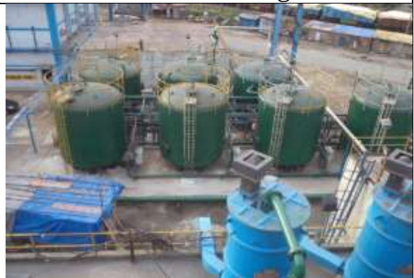
Side stream filter of CETP
