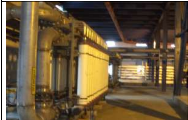
Reverse Osmosis Plant
