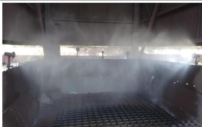
Dry Fogging System for Fugitive dust suppression
