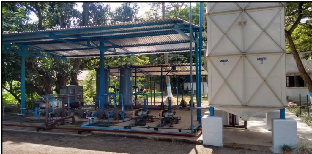
INSTALLATION OF 10 KLD SEWAGE TREATMENT PLANT (STP) FOR RECYCLING WATER DISCHARGED FROM CANTEEN & ADMINSTRATIVE BUILDING
