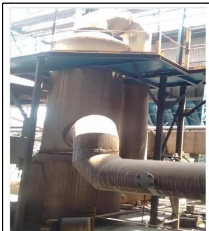
Fume Extraction System For existing Plant
