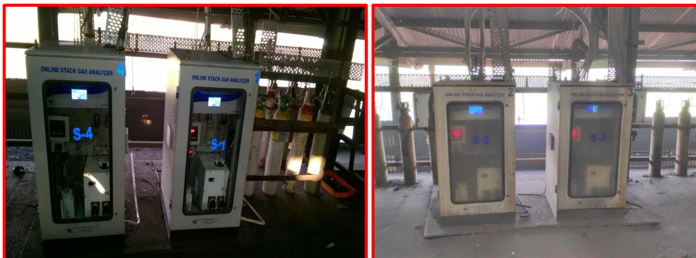
Continious Emission Monitoring System
