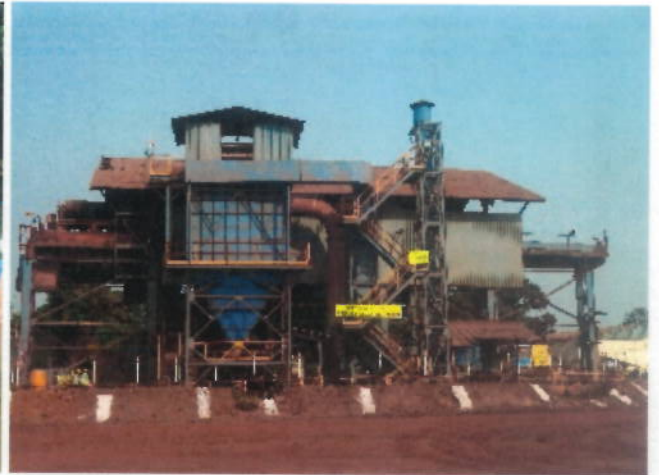
Dust Extraction System at Noamundi
