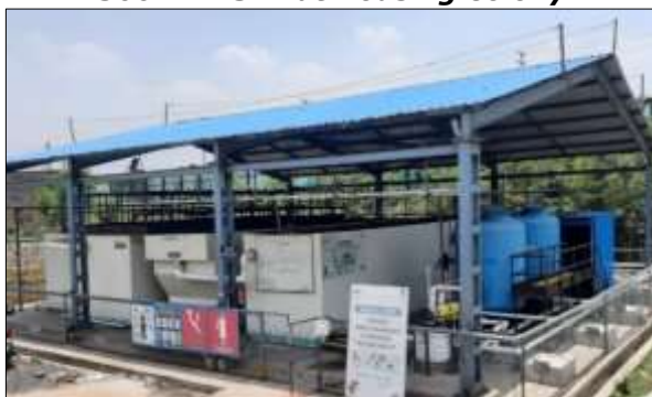
500 KLD STP at Housing Colony
