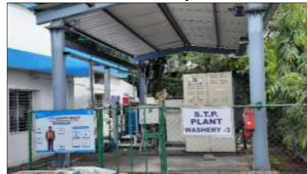
5 KLD STP at Washery-3 Canteen
