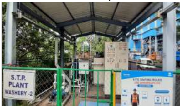
5 KLD STP at Washery-2 Canteen
