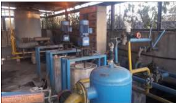
240 KLD STP at Mukundbeda Colony
