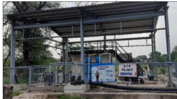
15 KLD STP at Chainpur Colony
