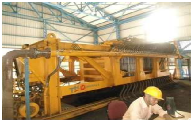
Mechanical tailings de-watering system
