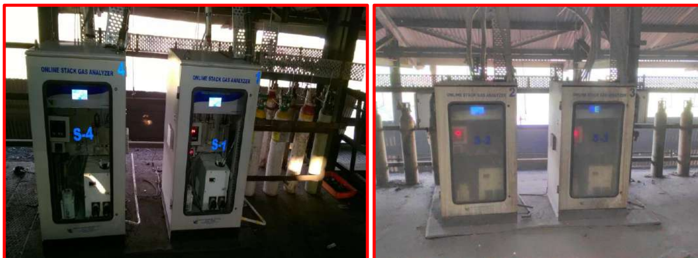
Continious Emission Monitoring System
