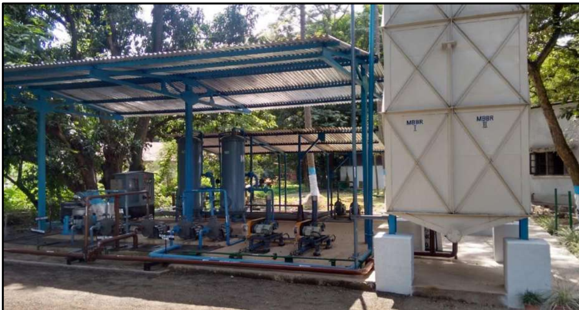
INSTALLATION OF 10 KLD SEWAGE TREATMENT PLANT (STP) FOR RECYCLING WATER DISCHARGED FROM CANTEEN & ADMINSTRATIVE BUILDING
