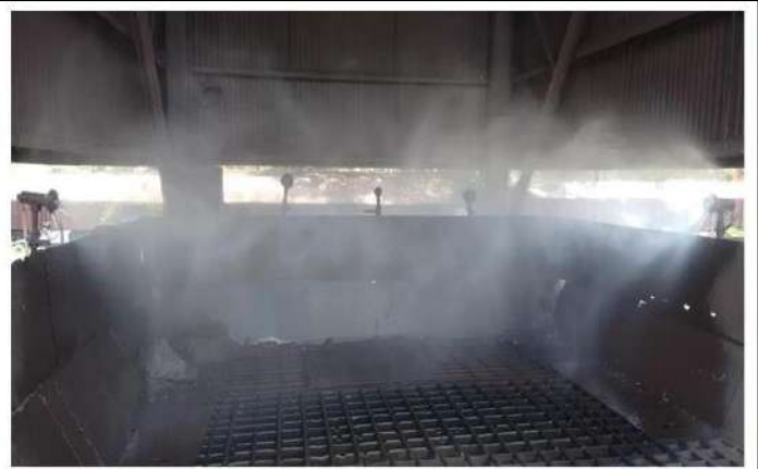
Dry Fogging System for Fugitive dust suppression
