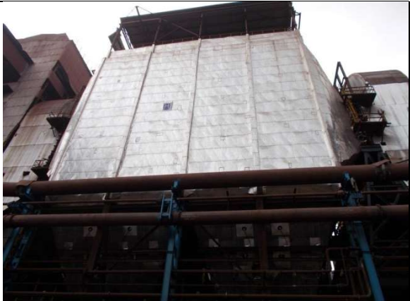
Sinter Plant 2 Waste Gas ESP
