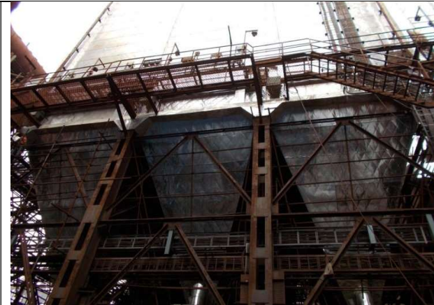
Sinter Plant 1 Waste Gas ESP
