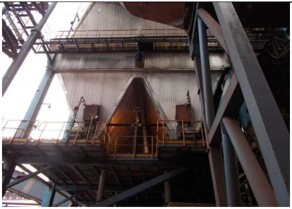
Sinter Plant 3 Refurbished ESP
