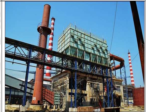
Stack: Bag Filters, ESP, Scrubbers & Cyclone
