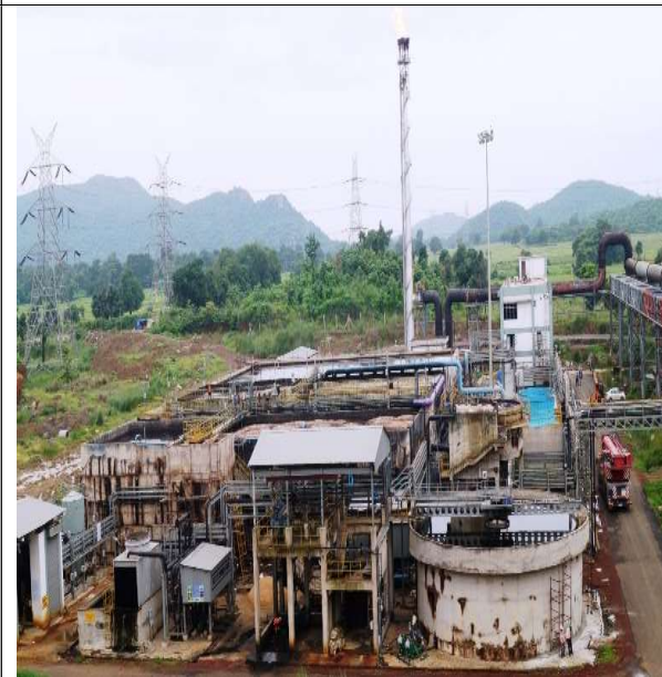
Process Effluent: Biological Oxidation Plant at Coke Ovens, Effluent Treatment Plants
