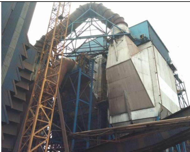
Sinter Plant 3 New Waste Gas ESP
