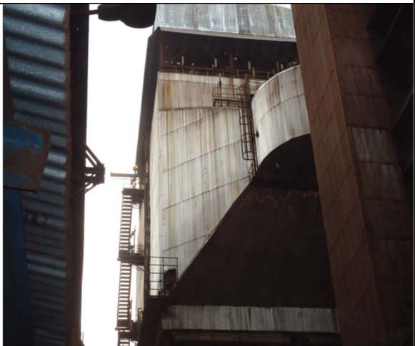
Sinter Plant 2 New Waste Gas ESP
