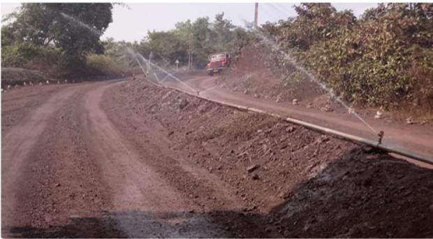
Fixed Sprinkling System
