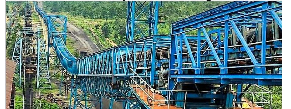
Long Pipe Conveyor at West Bokaro to reduce environmental footprint in coal logistics
