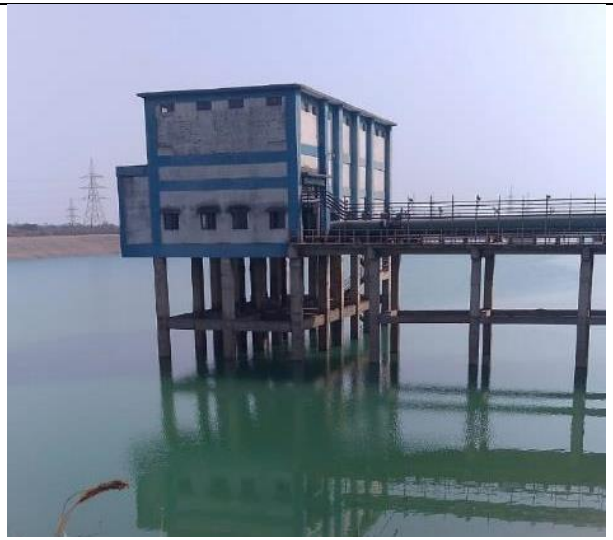
Water reservoir pump house inside plant
