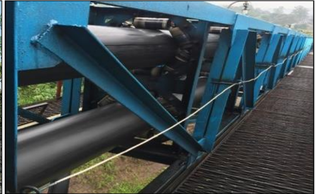
Pipe Conveyor for material transport
