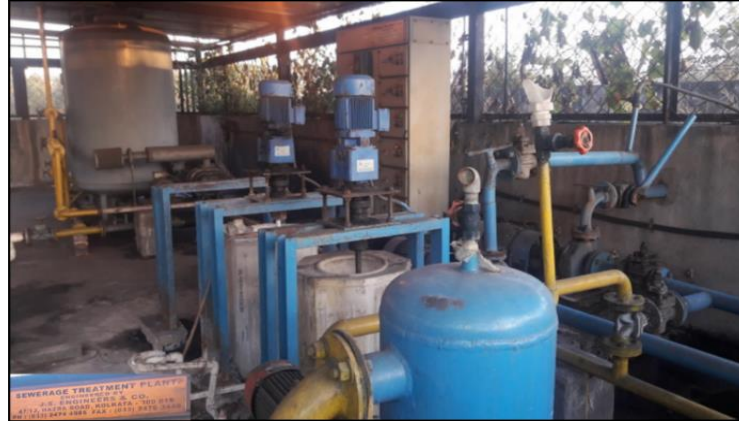
Sewage Treatment Plant (0.24 MLD) at West Bokaro
