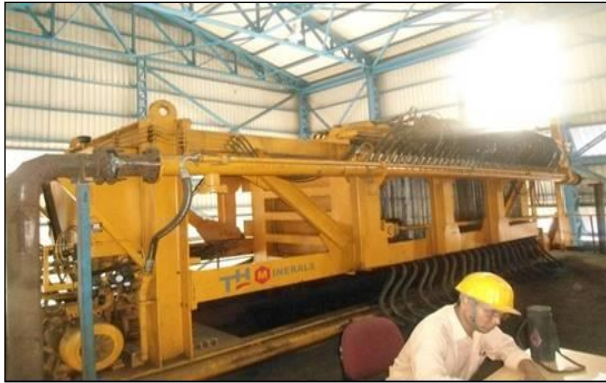
Mechanical tailings de-watering system
