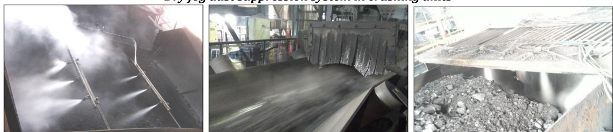
Water Mist Canon in coal stacking area
