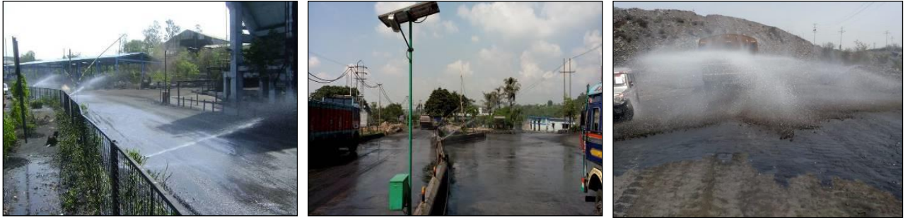
Use of fixed & mobile water sprinklers
