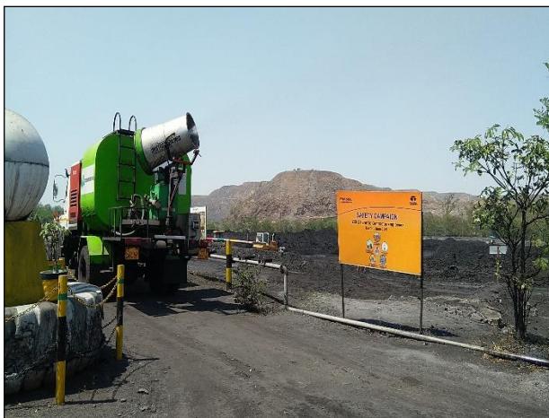
Water Mist Canon in coal stacking area
