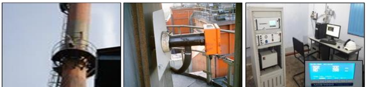
Continuous Emission Monitoring for Power House for PM, SO 2 & NO x data
