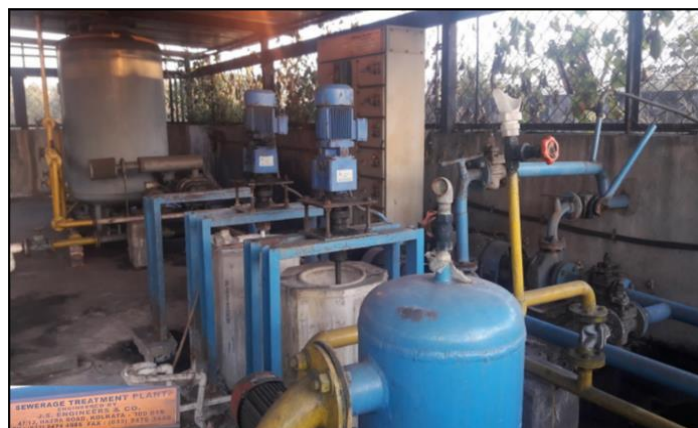
Sewage Treatment Plant (0.24 MLD) at West Bokaro
