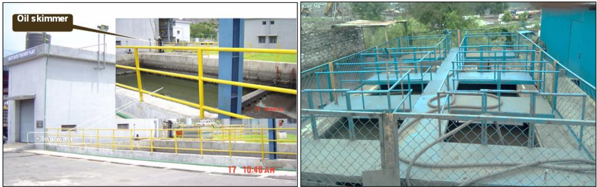
Oil & Grease trap at mines
