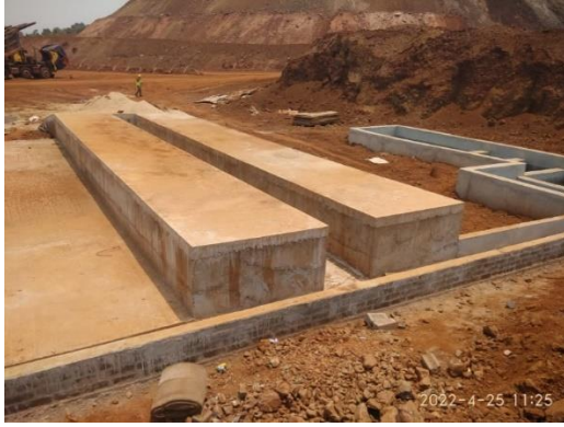
Vehicle washing with Oil & Grease separation pit
