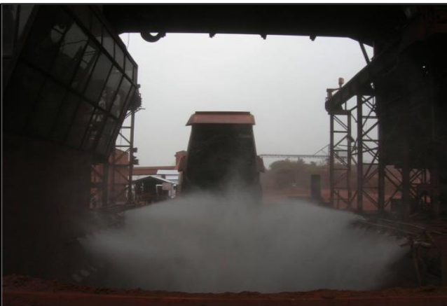
Water Jet System at Unloading Point
