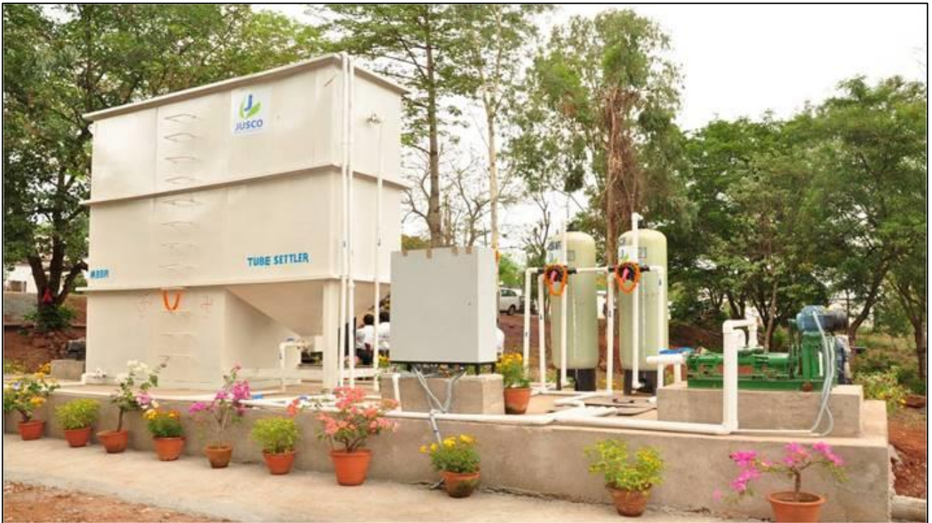
Sewage Treatment Plant
