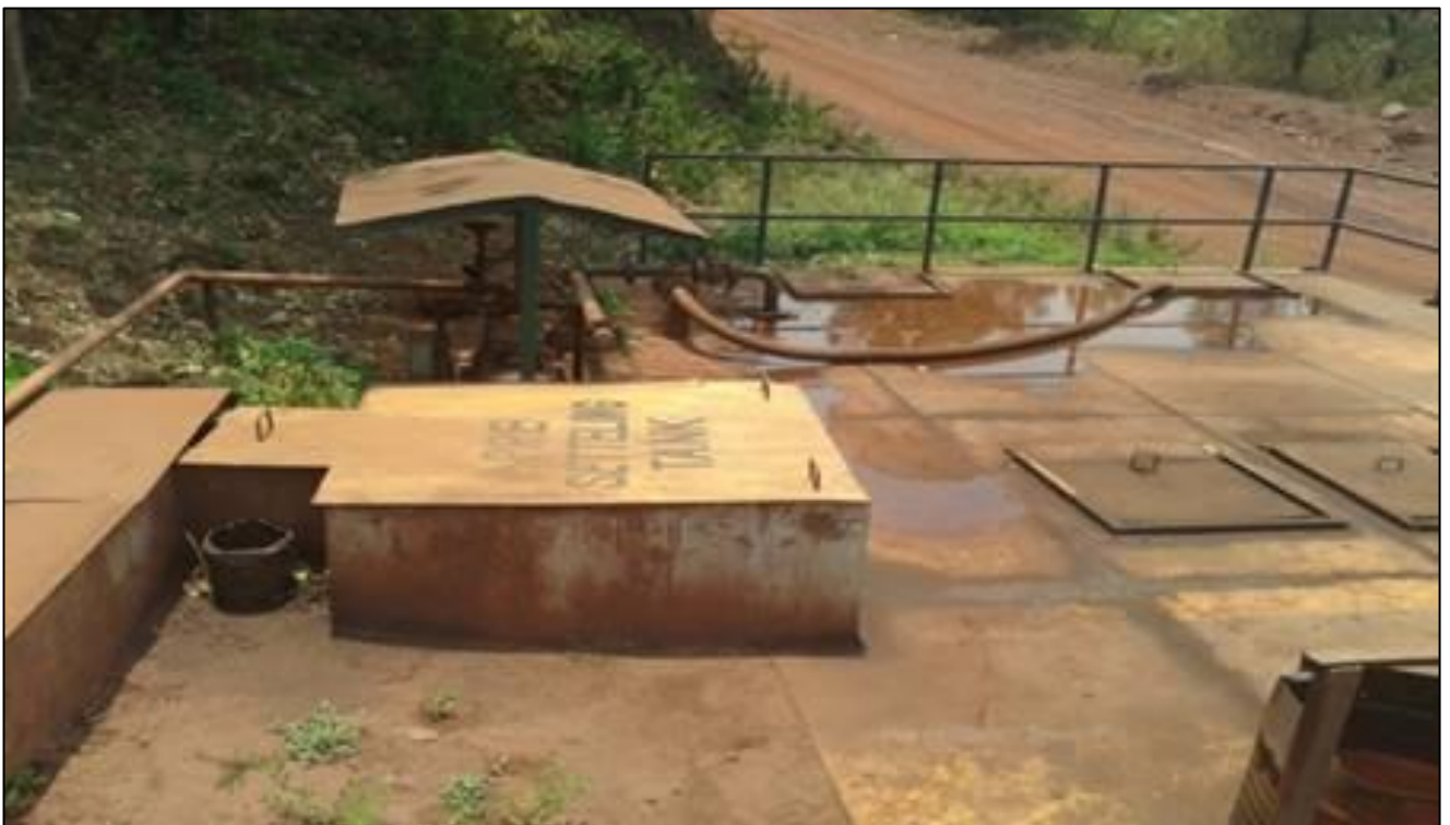
Oil & Grease Separation Pit
