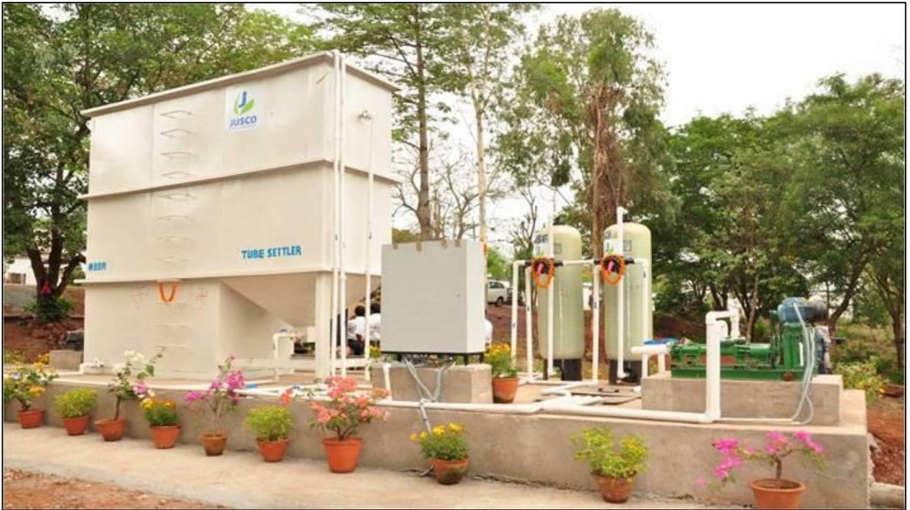
Sewage Treatment Plant
