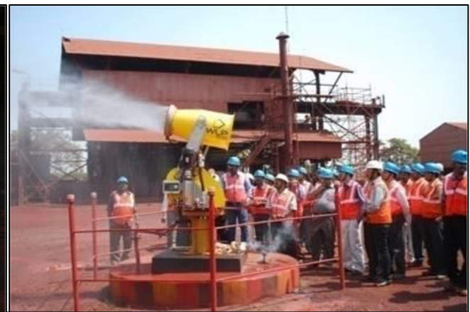
Water Mist System in Plant
