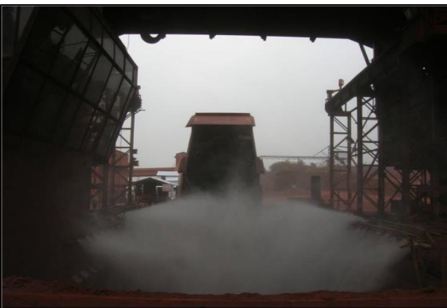
Water Jet System at Unloading Point
