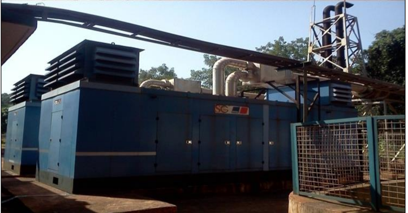
Acoustic Enclosures of DG sets
