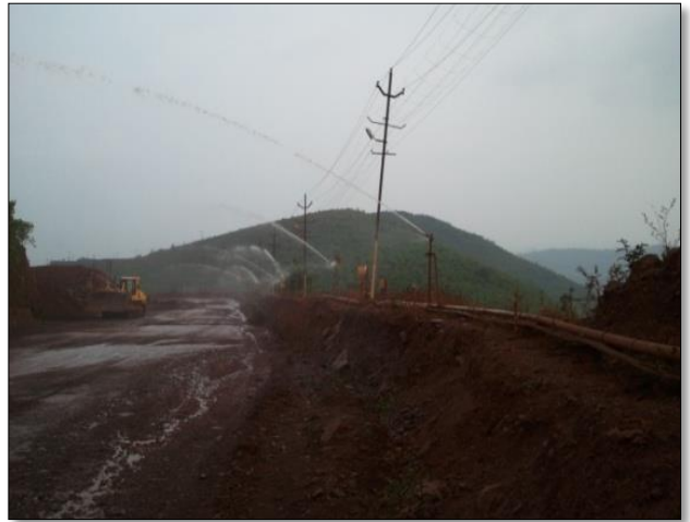
Stationary Water Sprinkler
