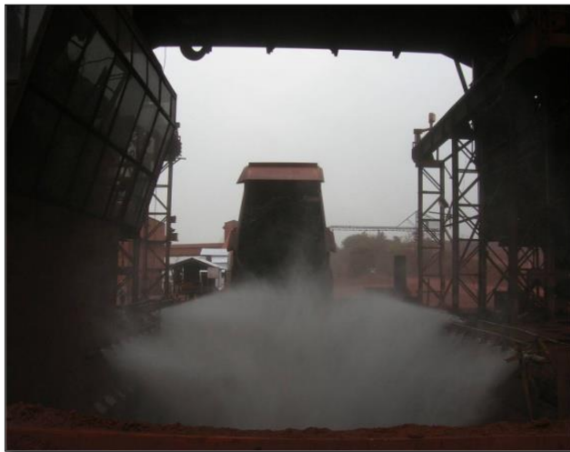
Water Jet System at Unloading Point
