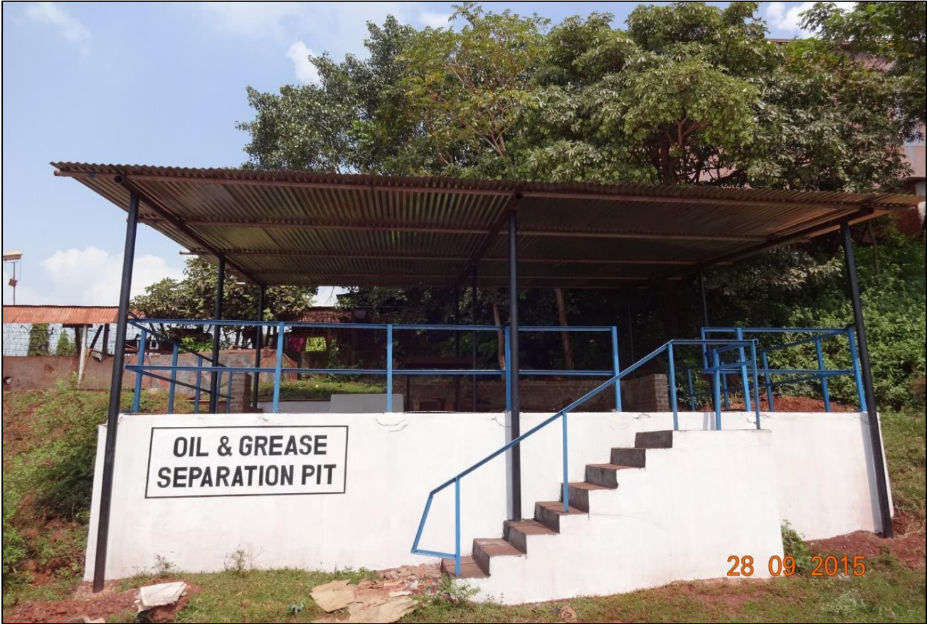
Oil & Grease Separation Pit
