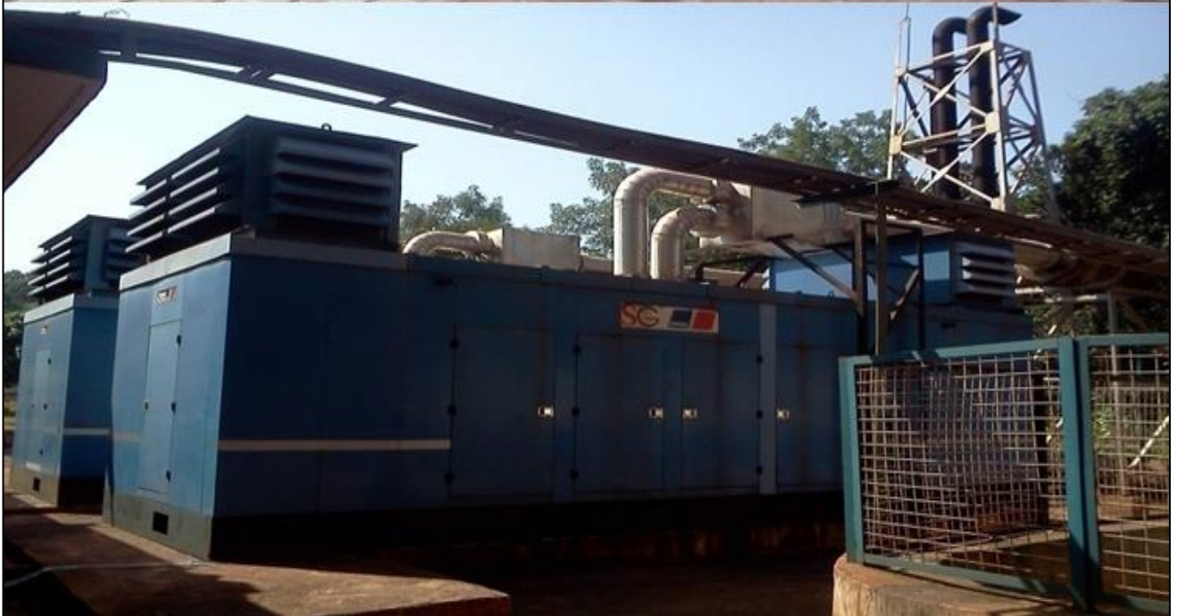
Acoustic Enclosures of DG sets
