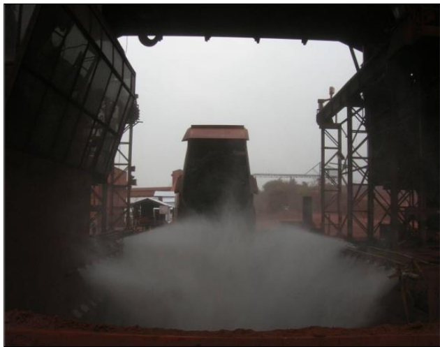
Water Jet System at Unloading Point
