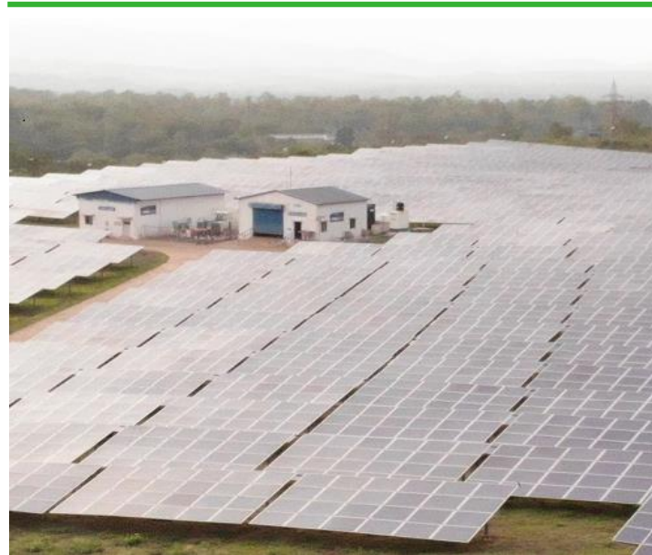
Solar park at Noamundi Iron ore mine
