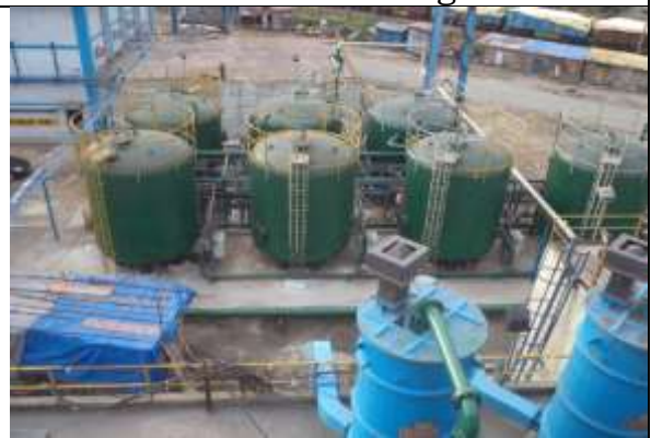
Side stream filter of CETP
