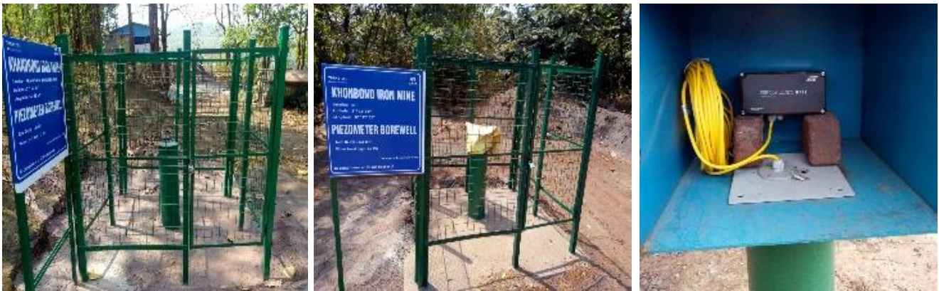
Piezometer (STP and Manganese) with digital recorder
