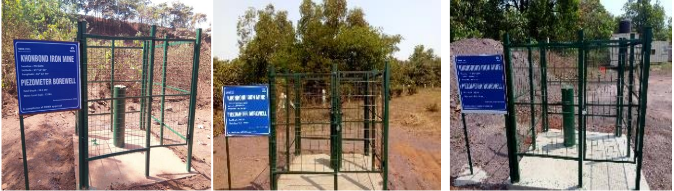
Piezometer (PB gate, Garden area, N orebody area)
