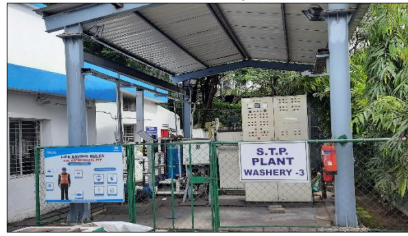
5 KLD STP at Washery-3 Canteen
