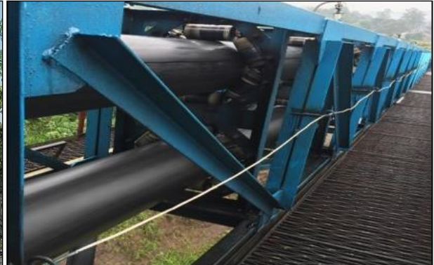
Pipe Conveyor for material transport
