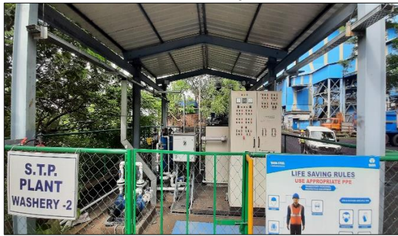
5 KLD STP at Washery-2 Canteen
