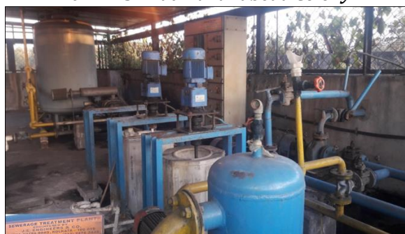
240 KLD STP at Mukundbeda Colony
