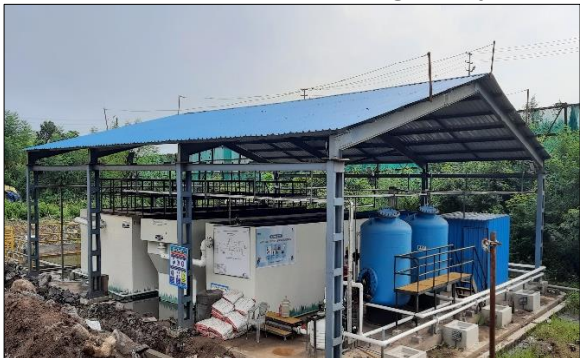
500 KLD STP at Housing Colony
