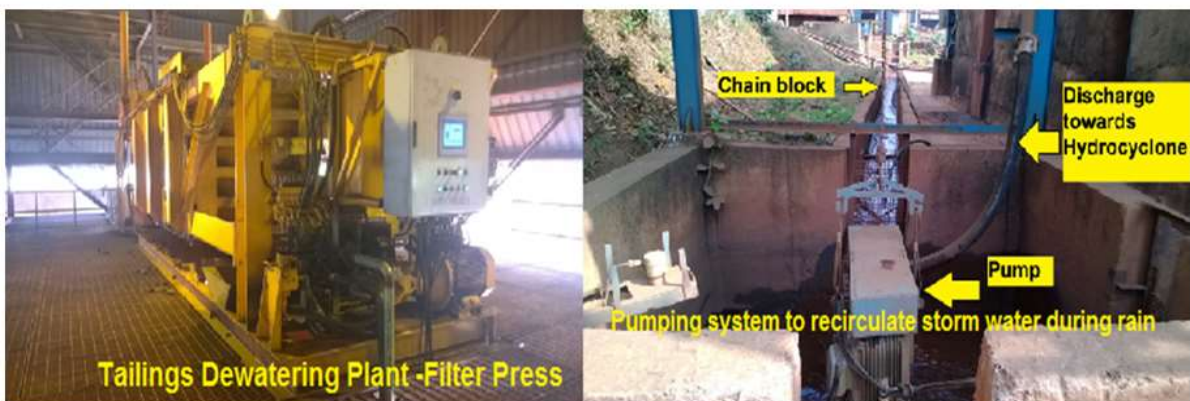
Tailing Dewatering Plant and Water Recirculation Arrangement
