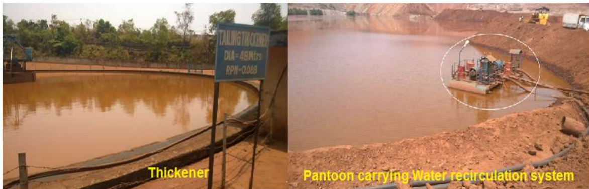
Thickener and Water Recirculation Arrangement
