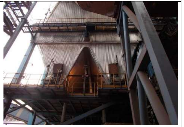
Sinter Plant 3 Refurbished ESP
