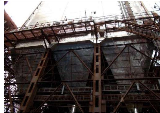
Sinter Plant 1 Waste Gas ESP
