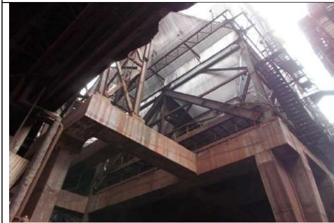
Sinter Plant 2 Refurbished ESP
