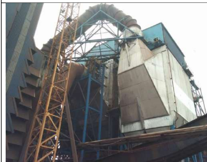
Sinter Plant 3 New Waste Gas ESP
