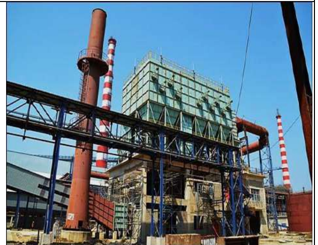
Stack: Bag Filters, ESP, Scrubbers & Cyclone
