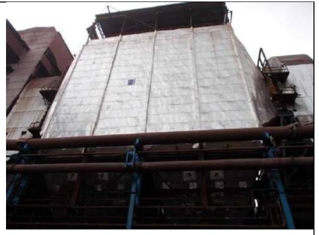
Sinter Plant 2 Waste Gas ESP
