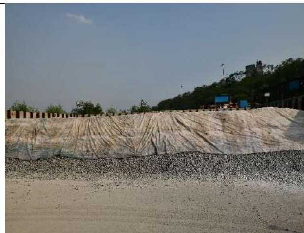
Open Steam Aging plant for LD Slag
