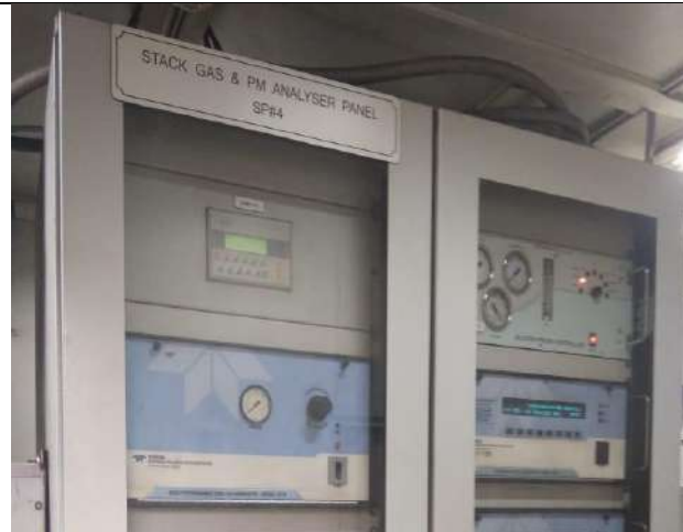
Stack Analyzers & Monitoring
