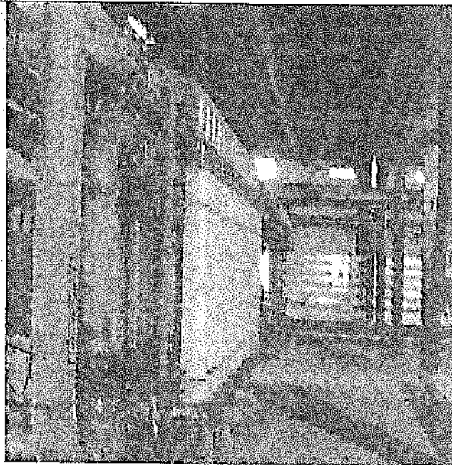
Reverse Osmosis Plant
