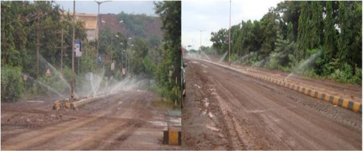
Stationary Water Sprinkler
