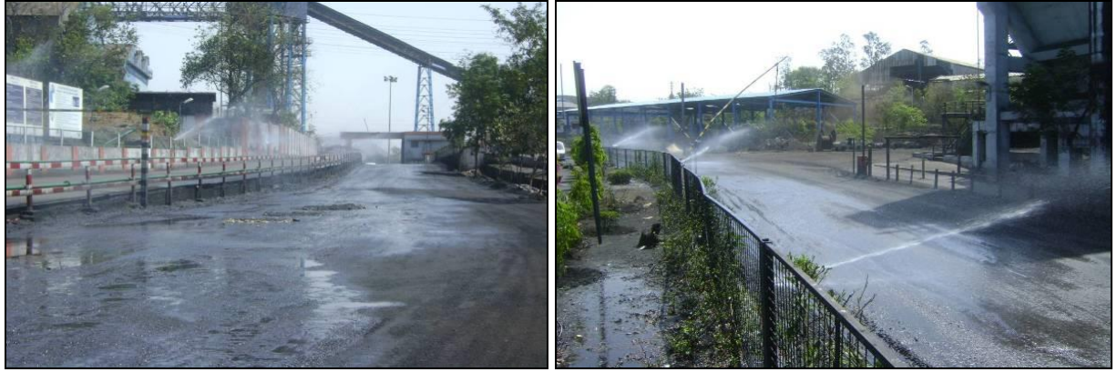
Fixed type water spraying system in Washery area
