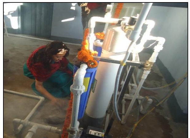
Water filtration system at Dhuni village
