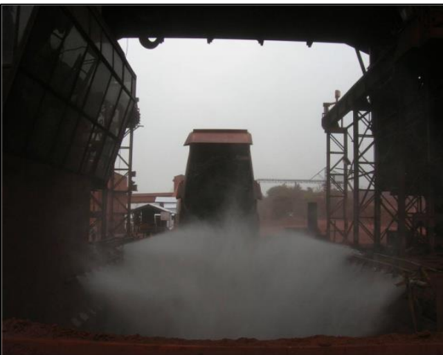
Water Jet System at Unloading Point
