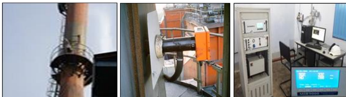
Continuous Emission Monitoring for Power House for PM, Sox & NOx data
