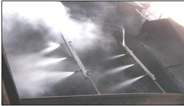
Dry fog system at CHP & crusher area
