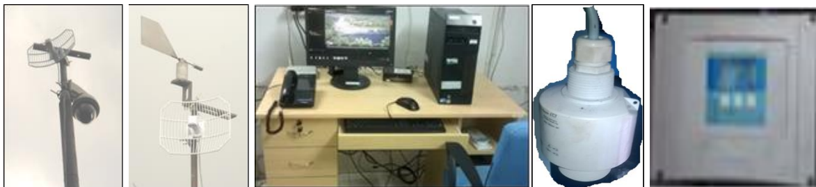
Online Effluent Monitoring System installed at site
