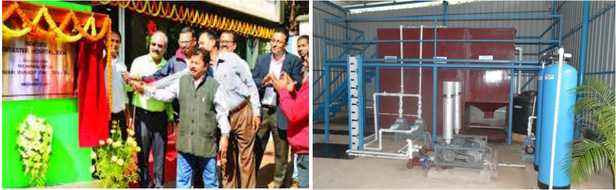
10 KLD Effluent Treatment Plant (ETP) at Tata Steel Hospital Joda (Dec 2017)
