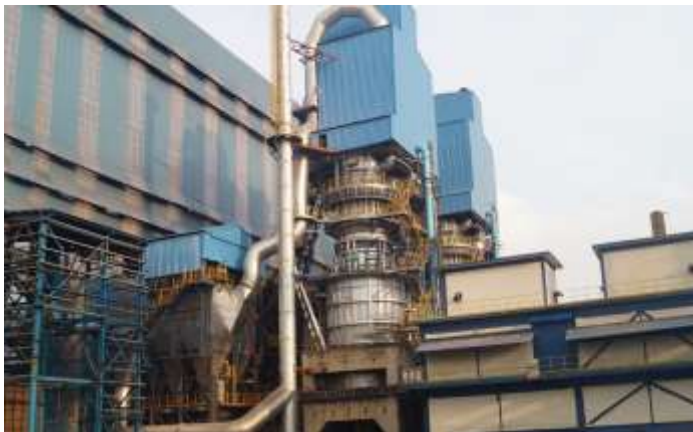
Lime Calcining Plant with Bag Filter
