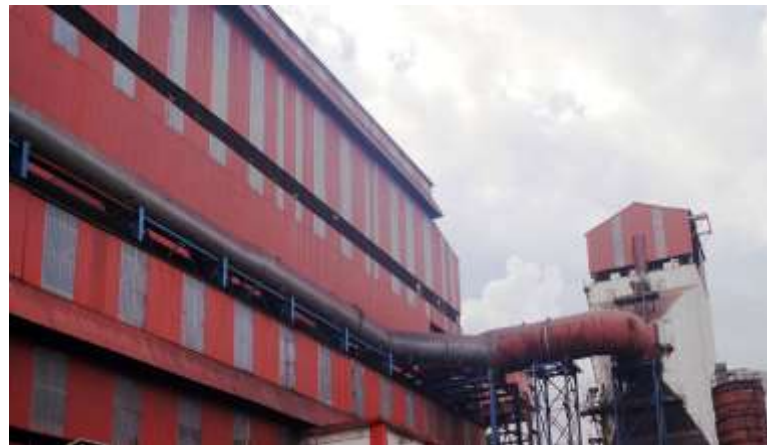
Dust Extraction System with ESP at Stock House of Blast Furnace
