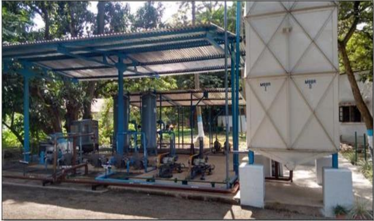
Sewage Treatment Plant Installed at FAP, Joda
