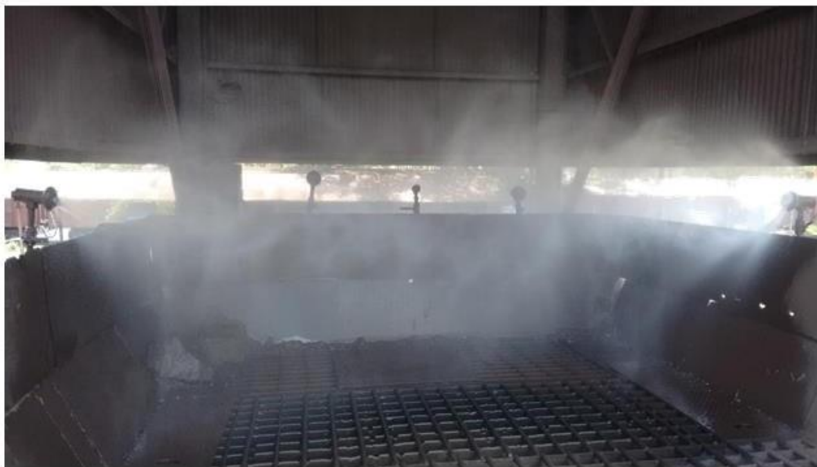
Dry Fogging System for Fugitive dust suppression
