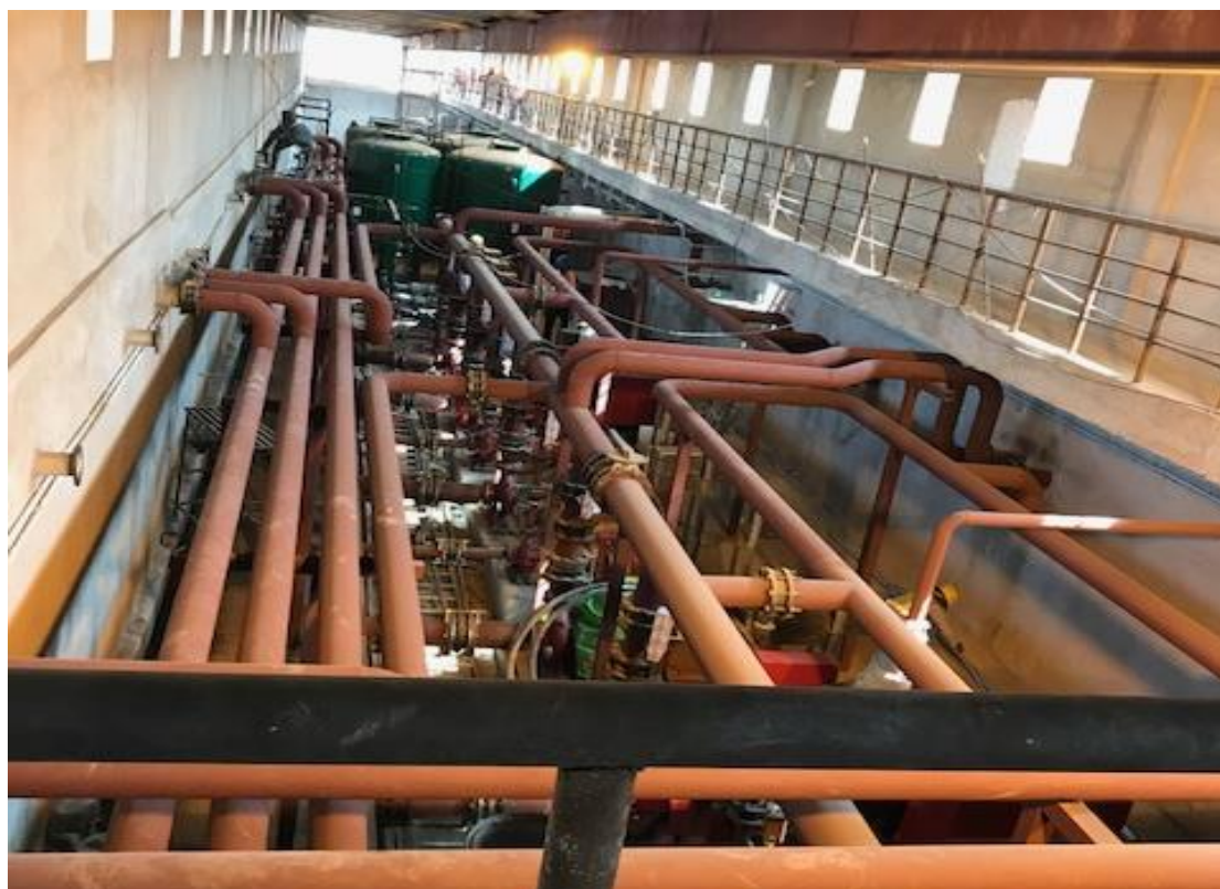
Water Treatment Unit
