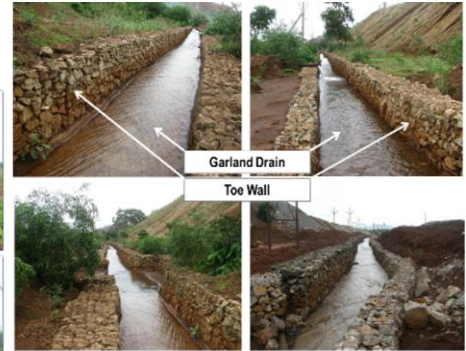
Garland Drains & Toe Walls
