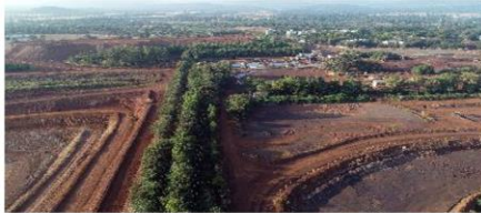
Back filling of mined out ore body II. It is planned to accumulate ~ 300 lakh cum of overburden which will save 60 Ha of land from degradation
